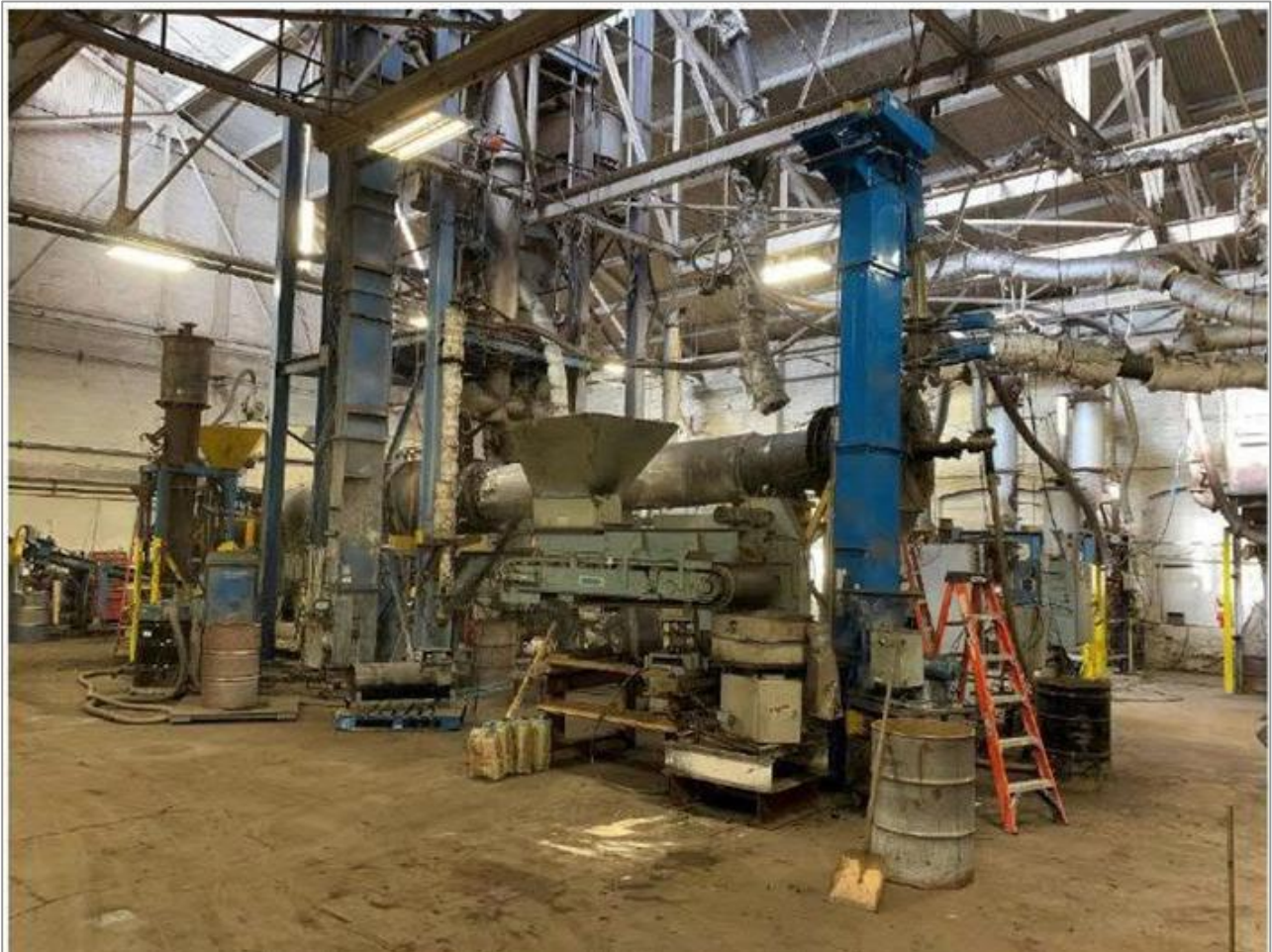
Figure 14.6 Pilot Plant Rotary Kiln, Feed-End to Right.
